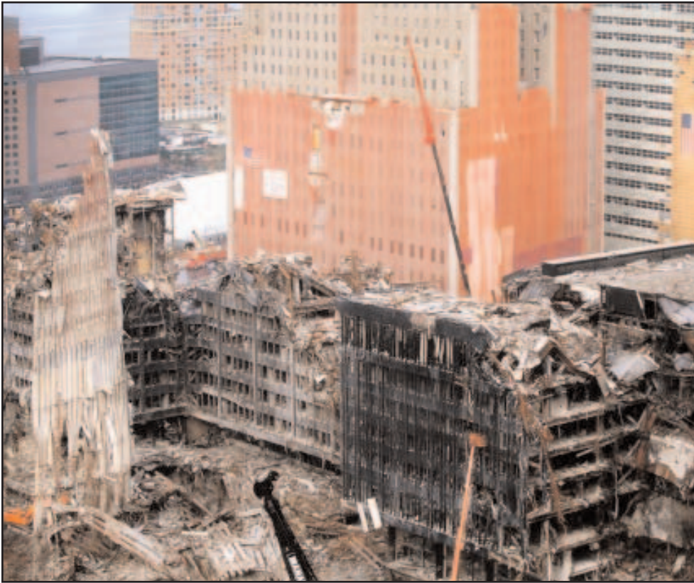
The rubble and remaining building structures of the World Trade Center are being broken down by heavy machinery. Manhattan, New York.
